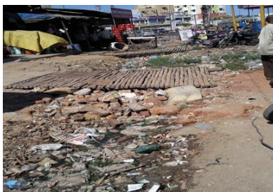
Figure.4. Poorly maintained drain in Medavakkam
